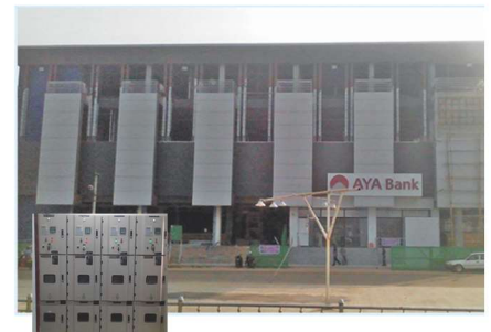
11/0.4 KV, 500 & 800 KVA Substation Ayarwady Shopping Mall (Patheingyi) Form Max Myanmar Co.,Ltd.
