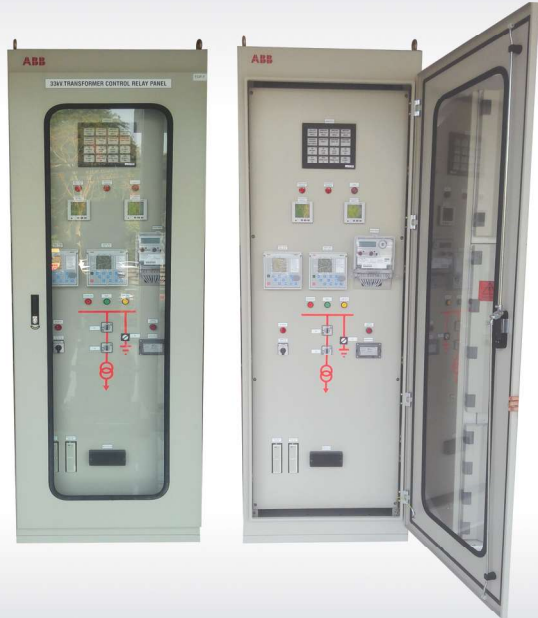
Control and Relay Panel
