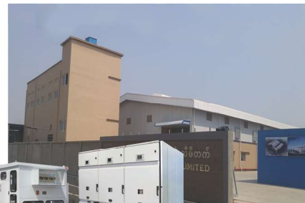
Harvey Handbags Factory 33/0.4KV, 2x1250kVA Dry Type Transformer & Substation Equipments
