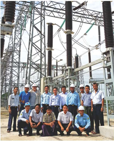
245kV Gas Circuit Breaker @ Pynmanar Substation
