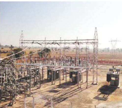
145kV Gas Circuit Breaker @ Magway Substation
