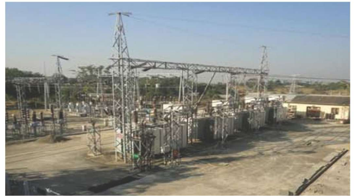
245kV, Gas Circuit Breaker @ Chauk Substation
