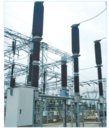
245 KV Gas Circuit Breaker (MEPE)
