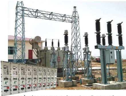
66/11kV,20MVA Substation @ Myo Thar
