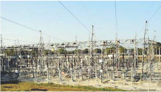
145kV Gas Circuit Breaker @ Thar Si Substation
