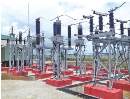
66/11 kV Myanmar International Port Substation
